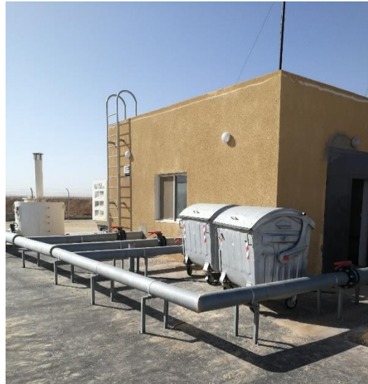
Figure 7. Wastewater pumping station in Za'atari, picture made by author
